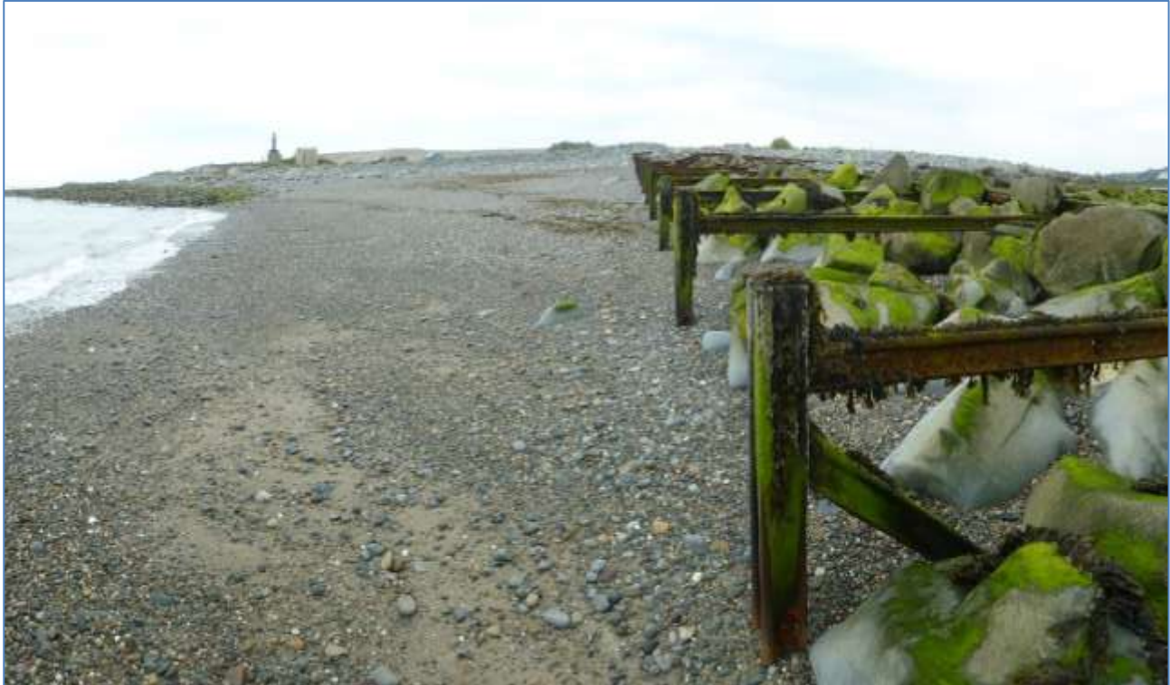
Plate 8: Missing side walings on updrift side of groyne
